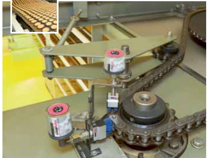
The drive chain of a transport belt, which allows rolls to cool, is cleaned with special blue brushes and lubricated with 2 simalube SL18 in 30 and 60 ml sizes.
